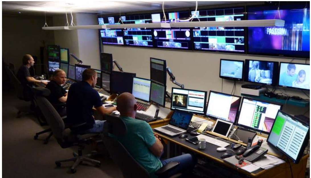
Right: Master control room at Ericsson Broadcast Services, Stockholm.
